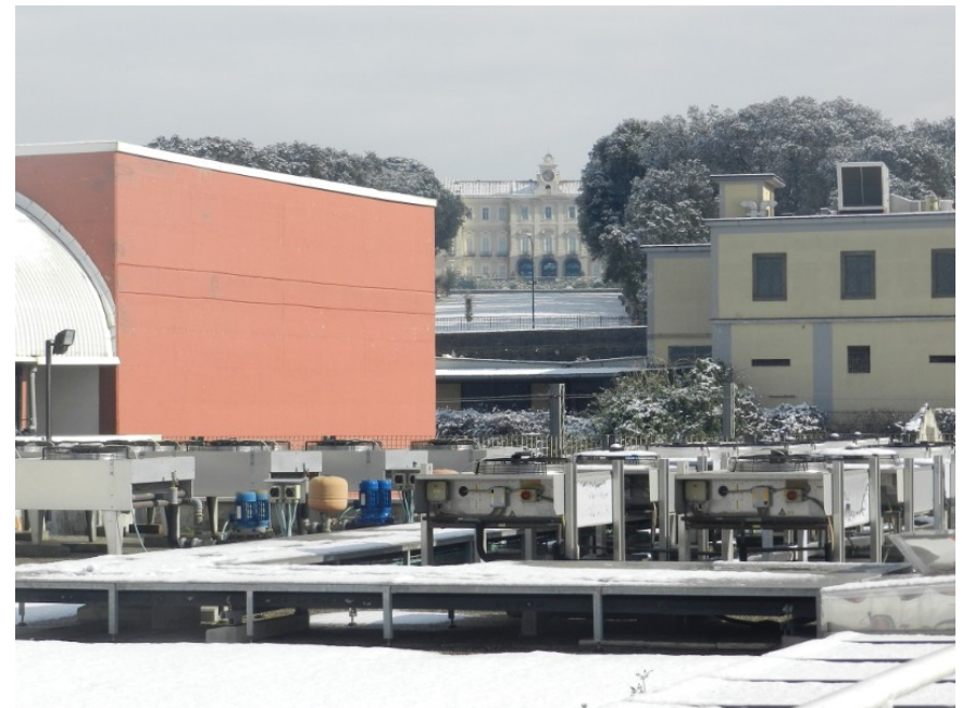
CRESCO clusters dry cooler system on the roof of the building, 27/2/2018
